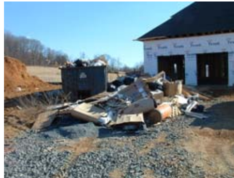
Debris at construction site
